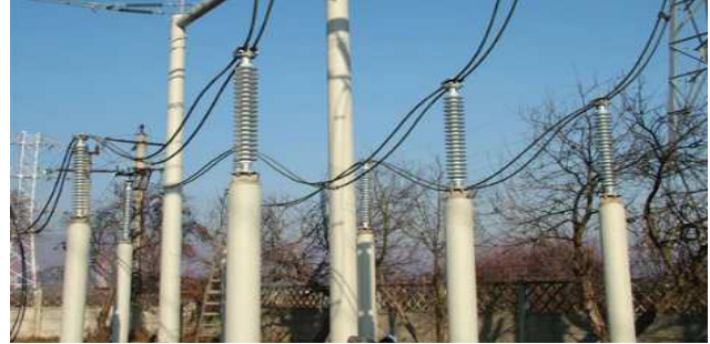
Fig 1.5: Showing the Post insulators
